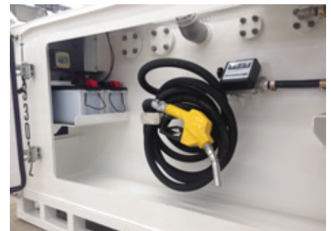
GENSET LINES AND PROVISIONS
